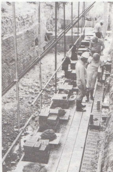
Peter Jones ( front ) directs work on replacing the brick face of Lock 9 on the Basingstoke. Original masonry face is being cut away, ( left ) Photo—R.H.P.
